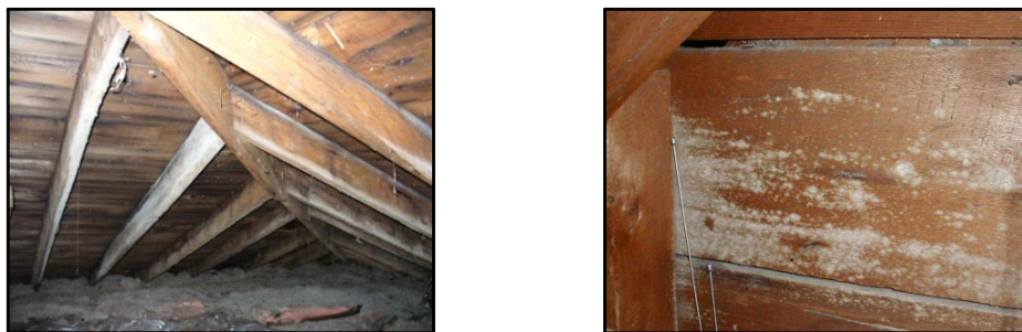
Figure 14 MOLD PRESENCE ON LUMBER
