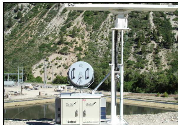
Figure 21 LRAD Corp. DEPLOYING LRAD® WITH AVIAN RADAR TO PREVENT WILDLIFE FROM ENTERING TAILING PONDS
